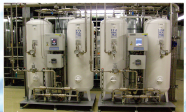
LARGE INSTALLATION IN HOSPITAL
